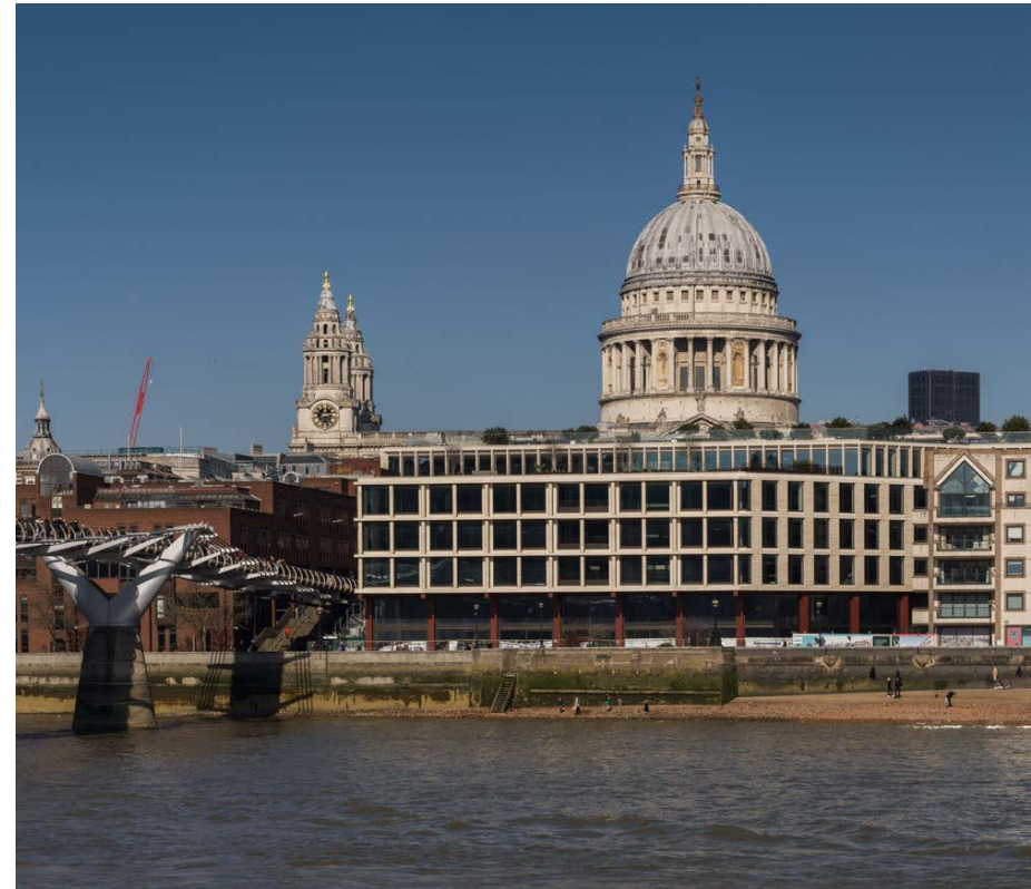
St Paul's from the south bank looking north to Millennium House under construction and now obscuring the view of the entablature or main body of the Cathedral (© Historic England Archive)
